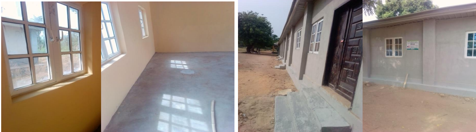
Completed wall and floor plastering, inside and outside painting, fixing of windows and doors
